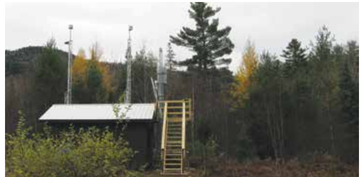
Air monitoring equipment installed at Huntington Wildlife Forest AMNet site in New York.
